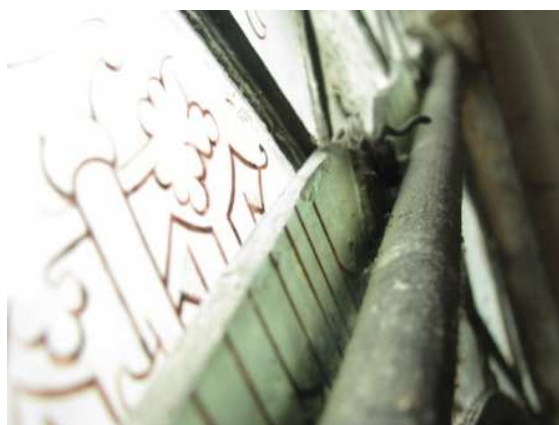
The crudely chopped upper edge of the internal panel. Note the two layers are touching.
