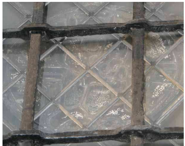
External surface with white corrosion deposits.
